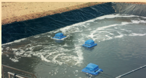
Turbo-Jet 1.1 kW – three aerators working in an oxidation-pond
